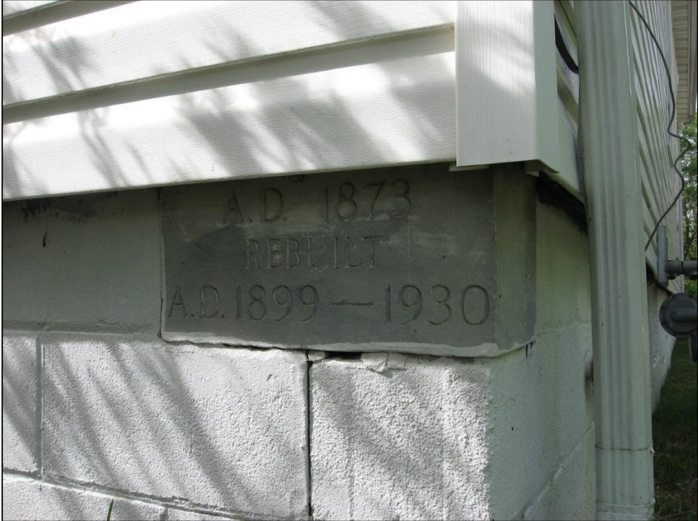
Above: A keystone on the front, right corner of the building announces its original 1873 construction date, along with later renovation dates. Courtesy of Janice Jay Young.
