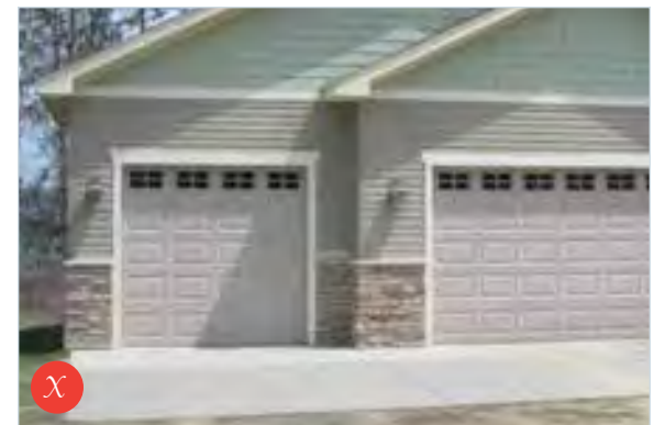
Garage door interrupting joint between materials and masonry is proud of siding above
