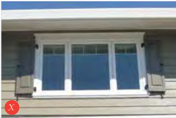
Shutters too small for openings
