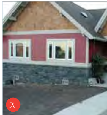
More than two materials on façade; masonry proud of siding above
