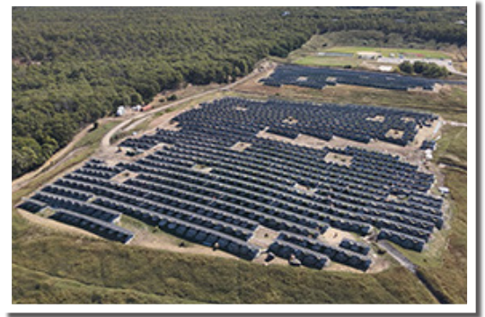
North Sea Solar Array, March 2025
